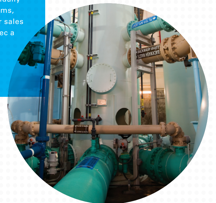
right: City of Litchfield Water Treatment Plant Litchfield, IL
