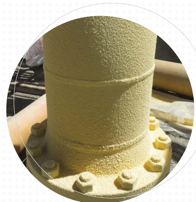
left and below: Refinery Piping Bakersfield, CA
