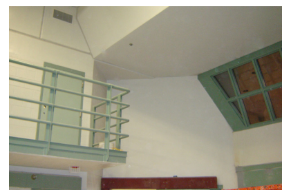
Tnemec coatings were used on both the interior and exterior of the North Branch Correctional Institution in Cumberland, Maryland.
